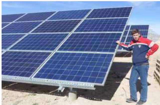
Figure II.40 : Station de production photovoltaïque Ain Imelh Msila
