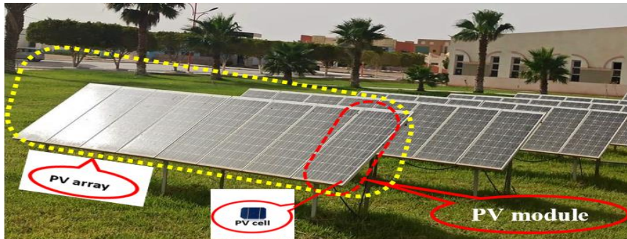
Figure 2.2. Photovoltaic (PV) field
