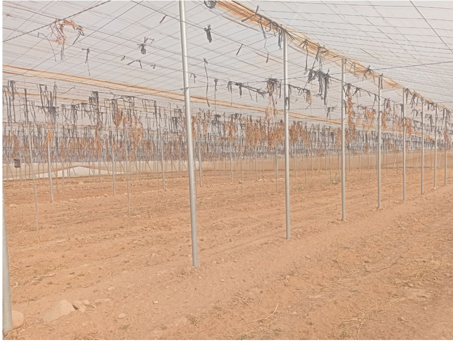
Figure 3.3: The 1-hectare commercial greenhouse at Branis site.
